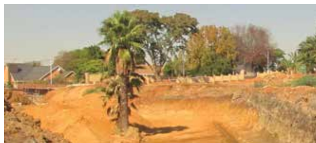
Existing trees are carefully re-located and on project completion indigenous trees will be planted throughout the complex
